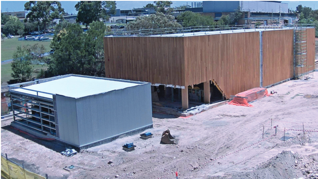
Figure 2. Construction status as of December 15th, 2014. Design of the main building minimises use of metal. Air conditioning, chilled water, electrical and compressed gas are supplied via service trenches from the plant building at lower left.
