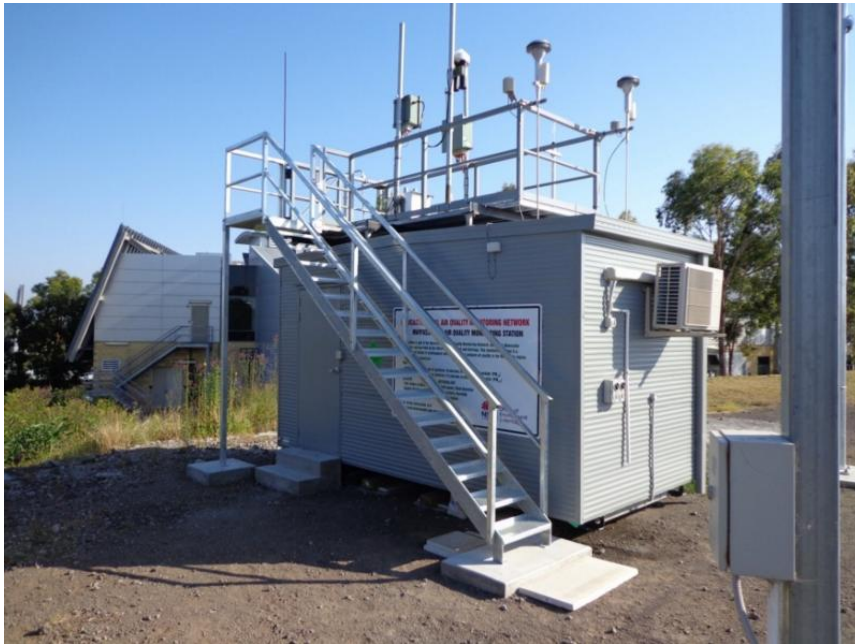
Figure 12: Mayfield Air Quality Monitoring Station located in the grounds of the CSIRO Energy Park
