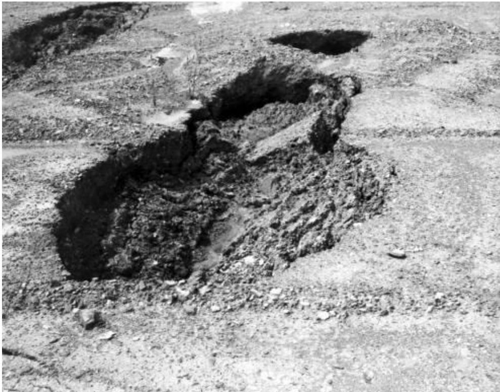
Figure 3. Subsidence over trenches in March 1969.
