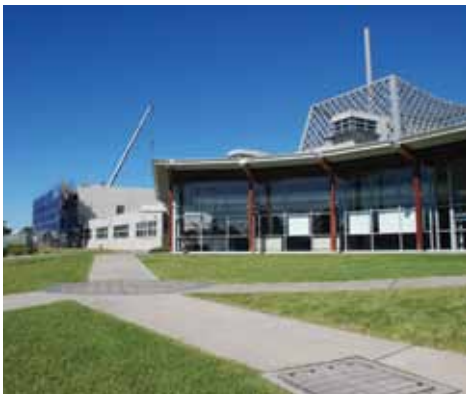
Construction of the OPAL building extension is well underway and expected to be completed by the end of 2012.
