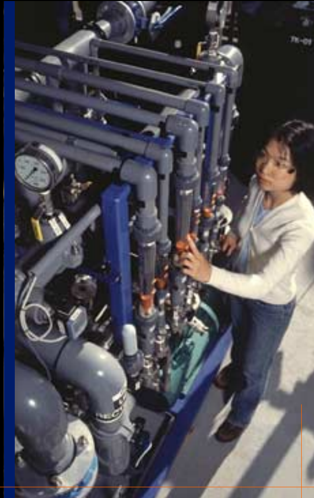
Chemical engineer Lynn Tan checks ANSTO's new water treatment pilot membrane plant. The pilot plant will be used in assessing the feasibility of using membrane technology to remove trace levels of radionuclides from low-level radioactive liquid waste streams at the Lucas Heights site.
