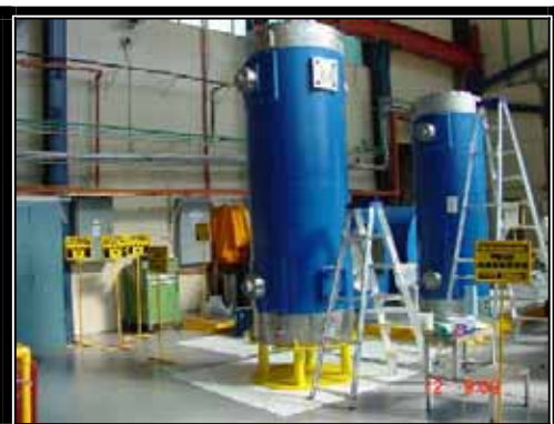
TN 7/2 Cask Loading Preparation Area
